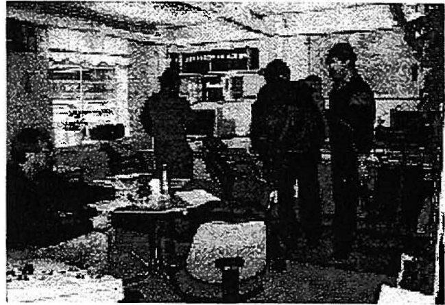
Picture 3: The control-room from which the computerised boiler is run also serves as a meeting-place.
